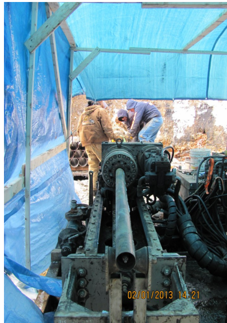
Above: Directional drilling into the mine pool at the Anna & Steve Gdosky Indian Creek Restoration Project
