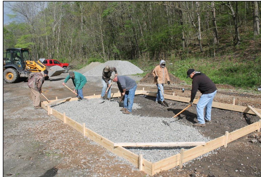
Volunteers installing a handicapped parking space at one of the trailheads for the Indian Creek Valley Trail.
