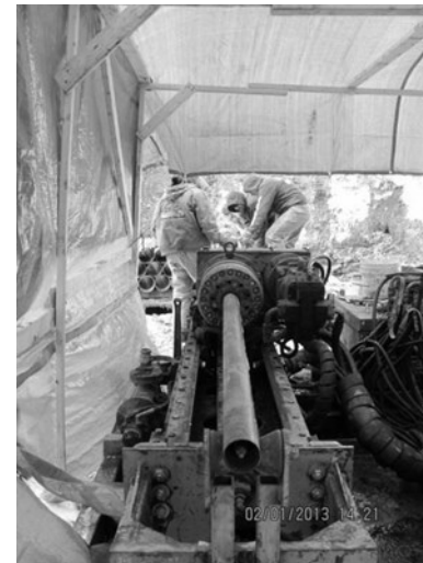
Above: A horizontal drilling rig was used to re-drill the boreholes into the mine pool
